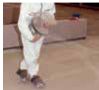
8. For a better bond, an additional wear layer is applied with Triflex ProPark and sprinkled with quartz sand.
