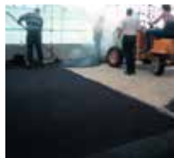
9. Just 3 hours later, hot mastic asphalt of up to 250 °C can be applied.
