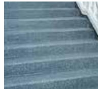
9. Apply the Triflex Cryl Finish 205 finish, blow in the Triflex Micro Chips, and it's done!
