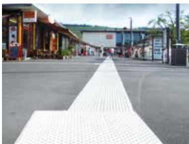
Railway station, Würzburg (DE) • Project: Station forecourt • Project size: 275 m ribbed marking • Systems: Triflex Tactile Marking, Triflex Precryo Cryl Cold Plastic 2K, Triflex Precryo Cryl Profile Plastic 2K
