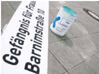
Women's prison, Berlin (DE) • Project: Pavement • Project size: 1,000 m 2 • System: Triflex Precryo Cryl Cold Plastic RP 2K
