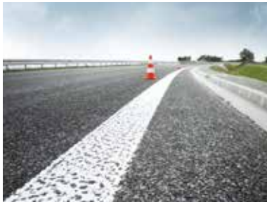
S3, Ostromice (PL) • Project: Trunk road • Project size: 6.1 km • System: Triflex Precryo Cryl Cold Plastic 2K
